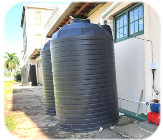
Water Harvesting - Immaculate Conception Convent (Kingston, Jamaica) The Mission Society funded water tanks for rain water collection to reduce dependence on the unreliable & expensive municipal water supply.
